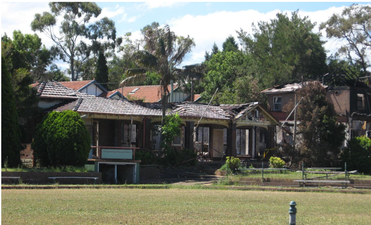
Figure 1 — northwards view showing fire damage including a burnt-out roof.
