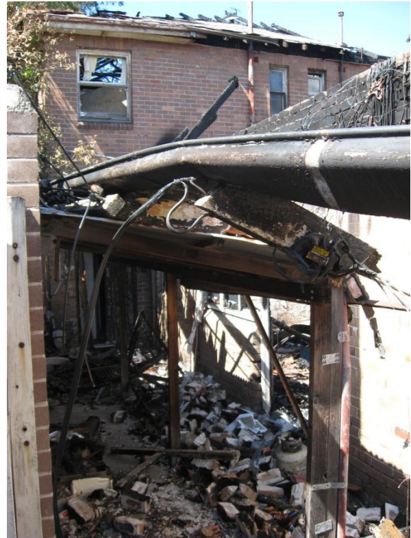
Figure 5 — north-east view between Bowlers Avenue store room (now collapsed) and the outside of Room 16.
